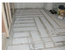
Above: One of the new art deco bathrooms, featuring black and white marble floors laid over The Floor Warming Company's electric UFH system, shown below
